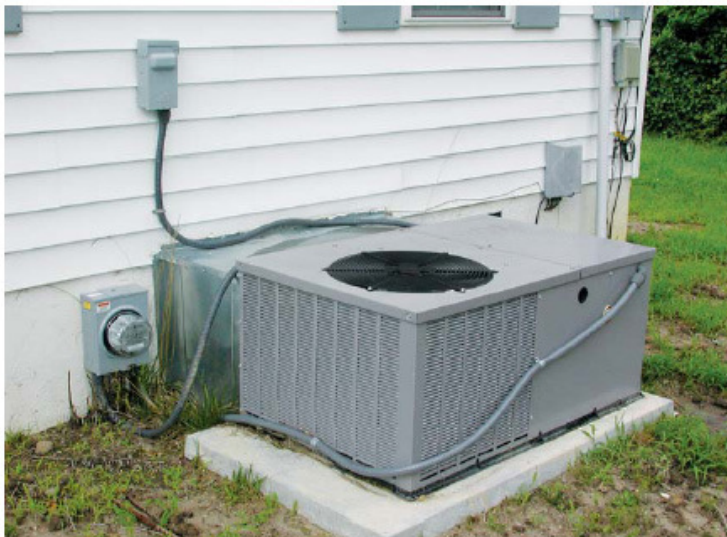
We outfitted all 12 houses with electricity submeters to record exact energy consumption by each home's package unit heat pump system.
