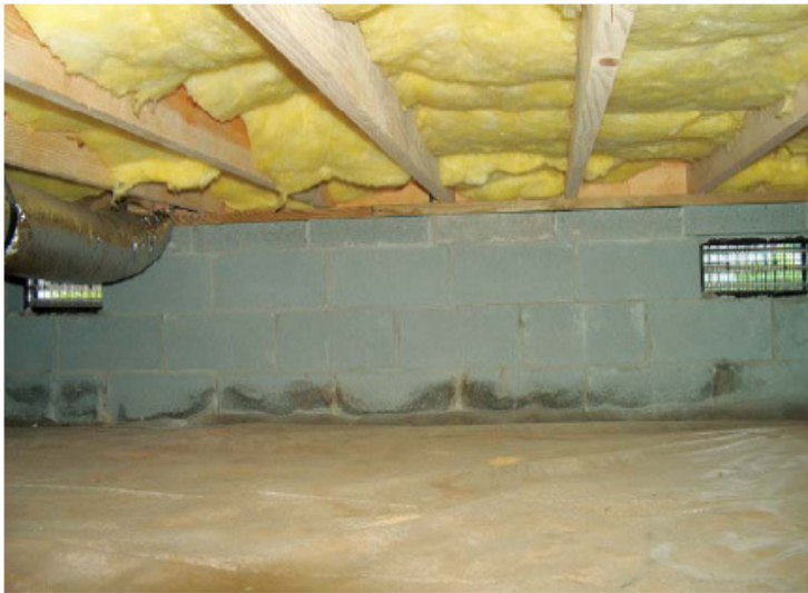
The wall-vented control houses in this study have much better crawlspaces than the typical crawlspace we encounter in the field. The control houses have well-installed insulation and 100% ground vapor retarder coverage of the soil, and no problems with intrusion of liquid water from outside.
