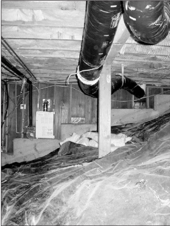
A poly barrier is being put in place to reduce moisture migrating from the soil surface.
