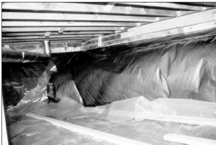
A well-sealed membrane installed in a crawlspace in Spokane, Washington, filled with soil air drawn from the highly permeable soil and by natural house depressurization. Exhausting air beneath the membrane solved this problem.
